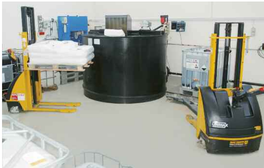
Production tank 8'000 liter
